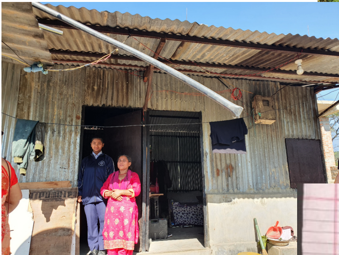
Left and above shows the zinc house & the surrounding area in November 2022.
