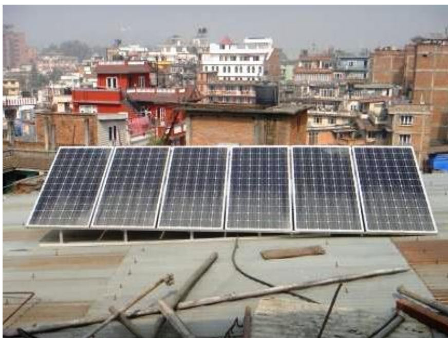
Shree Neel Barahi Upper Secondary School – Solar Panels for Computer Room
